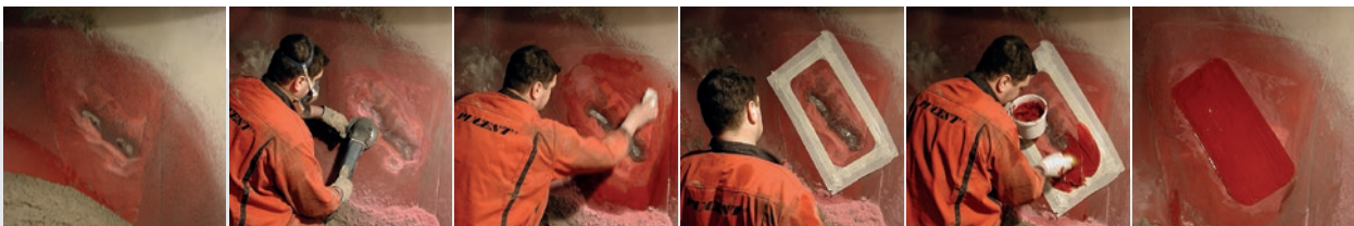
Damaged position... grind off
