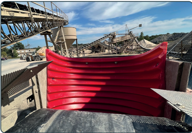
SZ panels bolted in the impact area of a conveyor belt.
