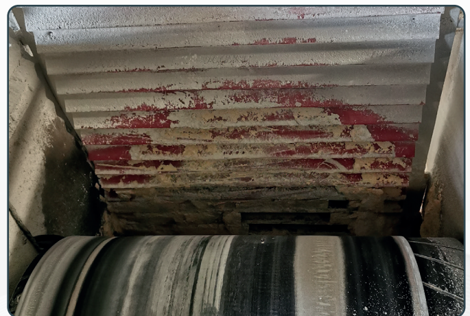
SZ panels semi-hanging in the impact area of a conveyor belt
